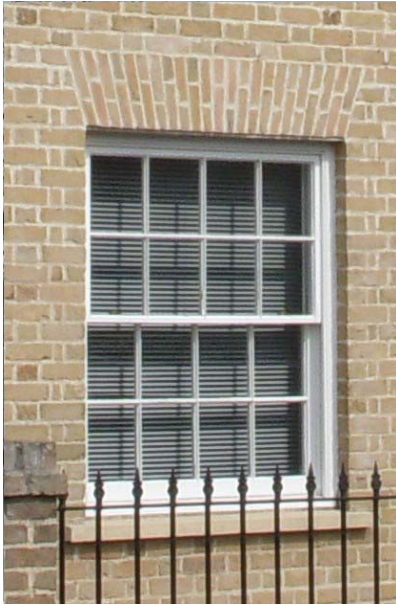
Traditional timber sash window to a new house set 100mm back from face of the brickwork and with a sub-cill. Note also the use of Flemish bond in the brickwork together with the shaped 'voussoir' bricks over the opening.
